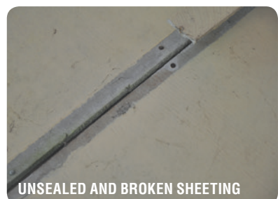
BROKEN ASBESTOS CEMENT SHEETING
