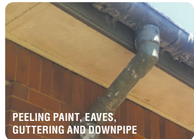
EXTERNAL PEELING PAINT EXPOSED TO WEATHER
