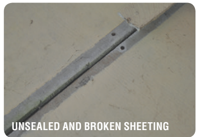
BROKEN ASBESTOS CEMENT SHEETING
